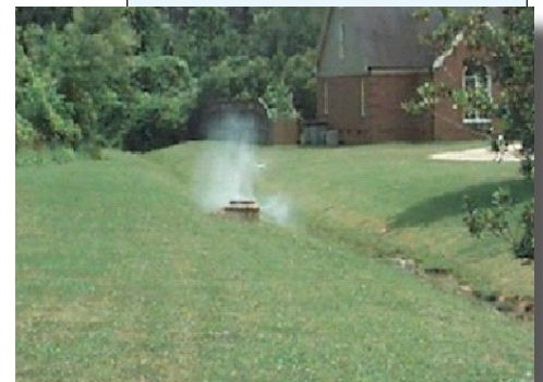
Smoke exiting the sewer system
